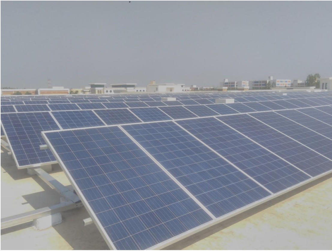
100KW Solar Power Plant Located at Rooftop of SIEM, Nashik
