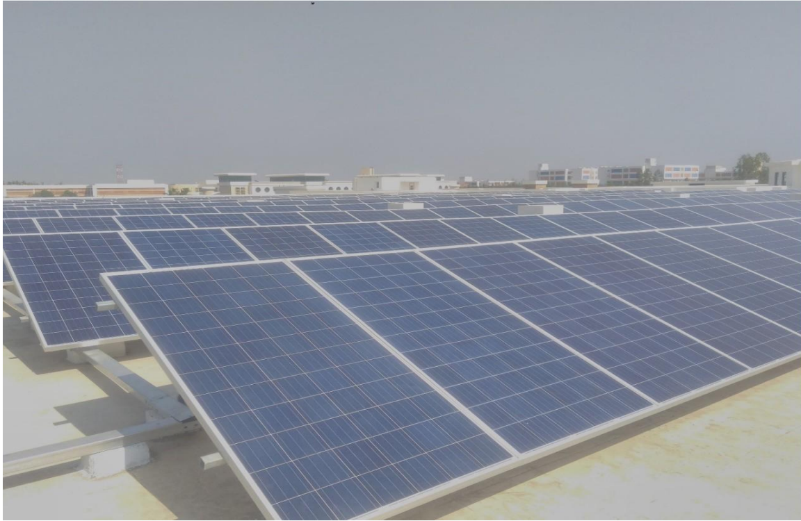
100KW Solar Power Plant Located at Rooftop of SIEM, Nashik
