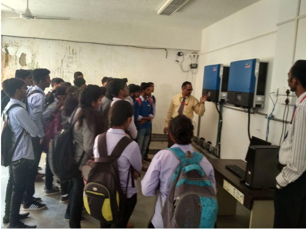
Prof.H.R.Kulkarni explaining the Real Time Monitoring of Plant to Students
