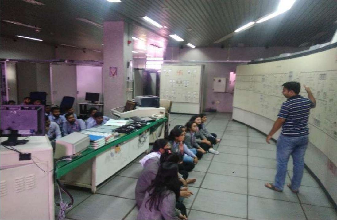
Dy. Engineer, Sunil Shenava explaining Single Diagram and Power Flow to Students
