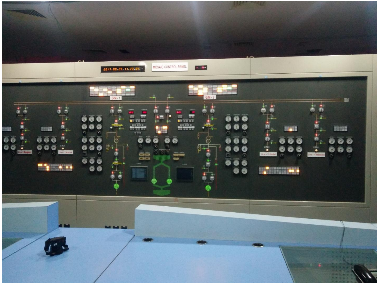
Control Panel Room at Ghatghar Hydro Power Station
