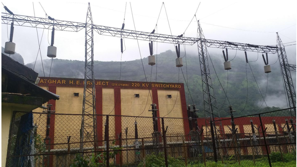
220 KV Switchyard at Ghatghar Hydro Power Station
