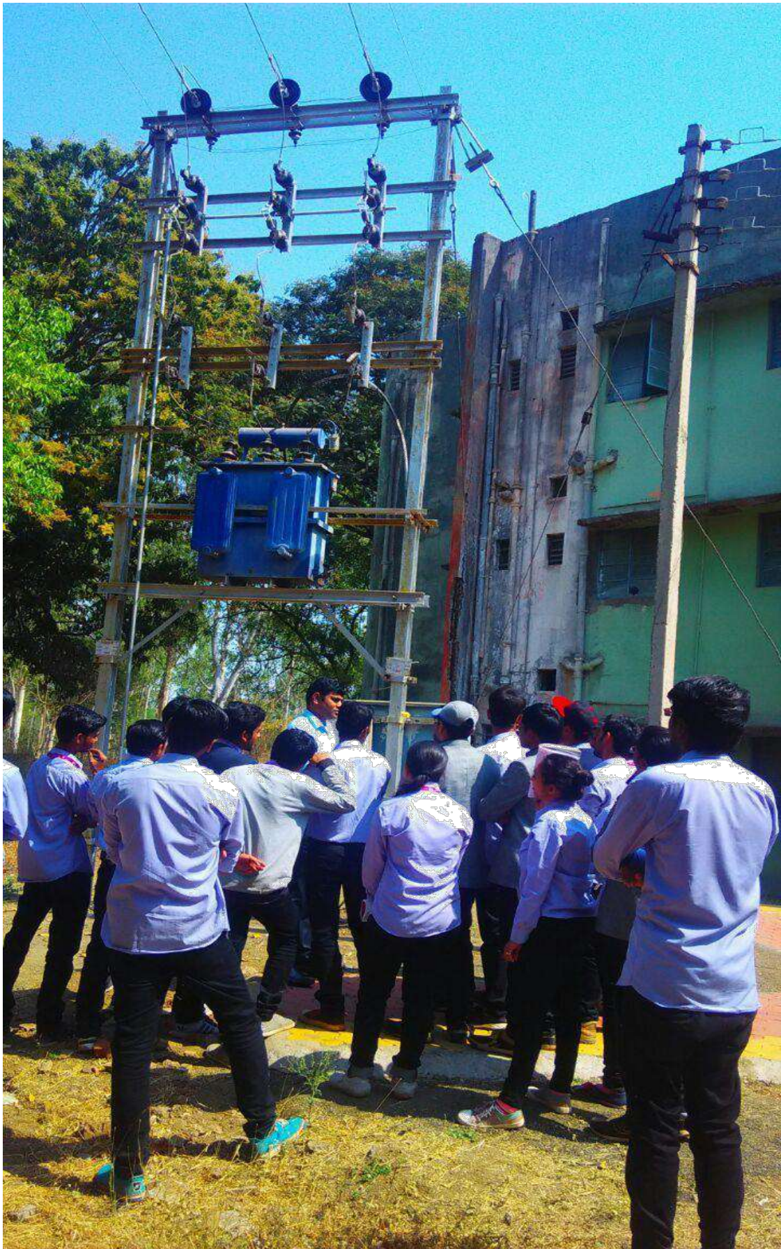
Er.S.Patil Demonstrating various equipment used in Distribution Transformer Centre.
