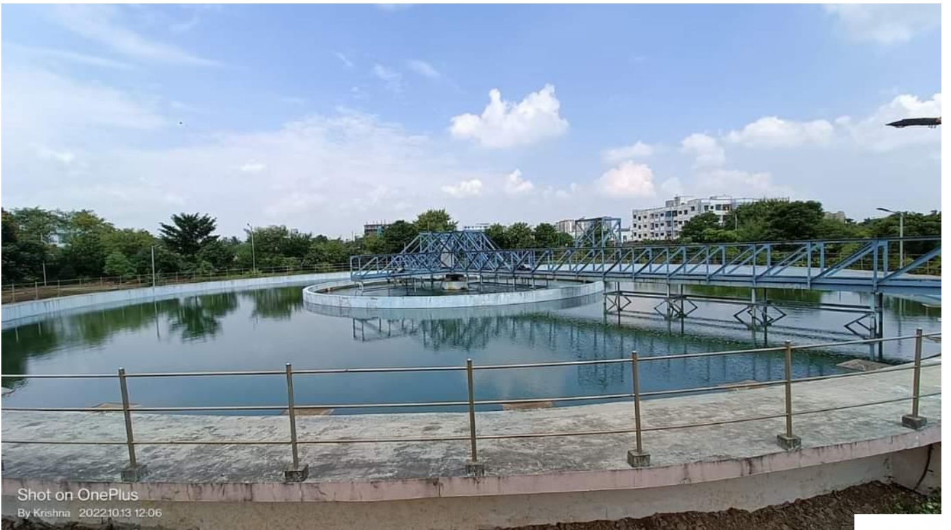
Clariflocculator View at Nilgiribaug WTP
