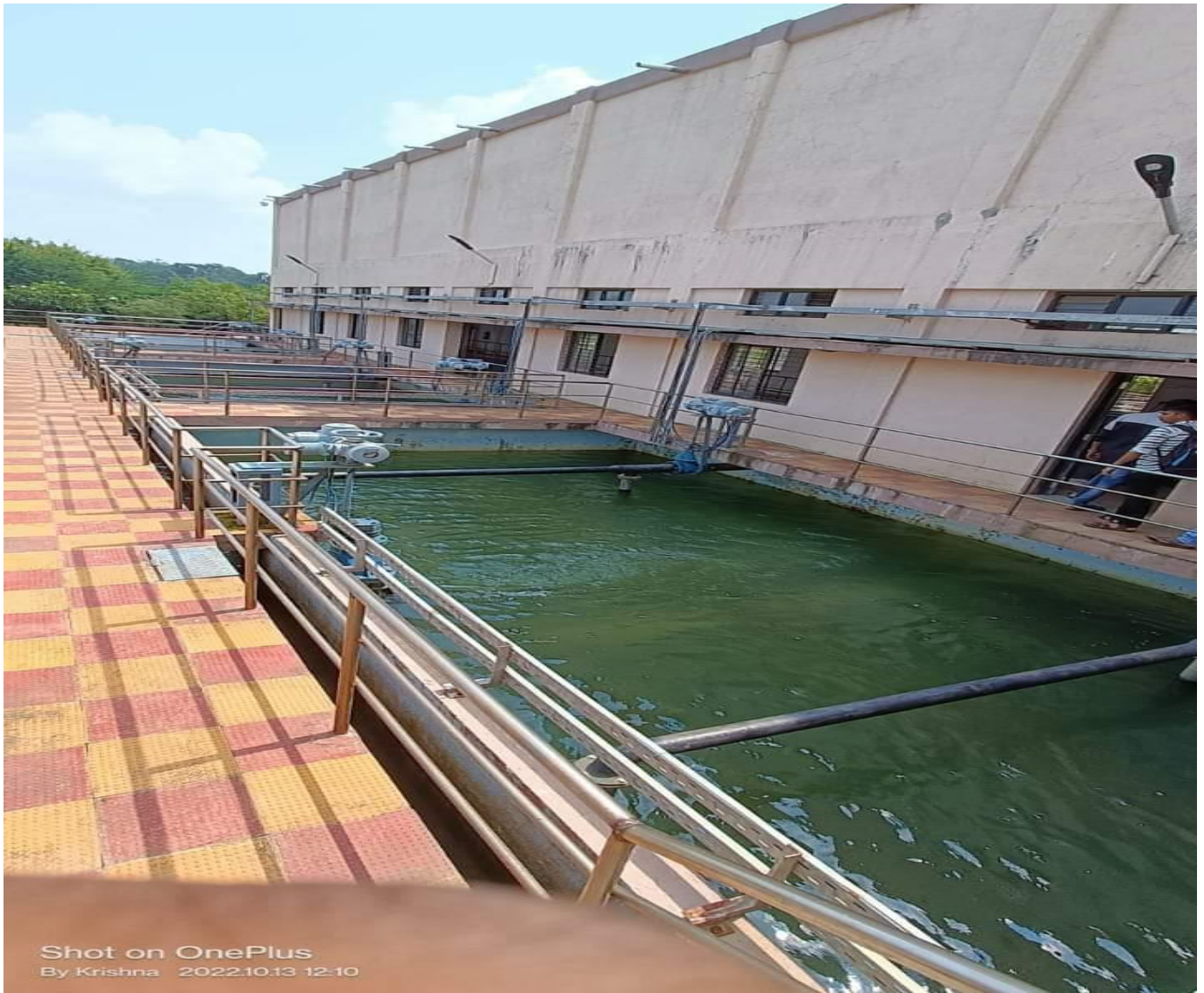
Rapid Sand Filter Under Regular Opearation
